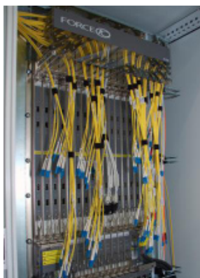
DE-CIX edge switch #8 provides additional 56 line rate 10GE ports for customer connections
